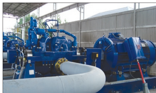
Obr. 7. Pohony s motorem 1 425 kW, 6 kV, 50 Hz
